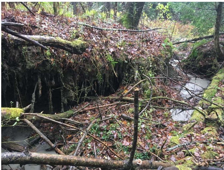
Figure 3. Failing gully bank, with accumulated sediment and debris in the channel in foreground; gray-colored runoff in background.
